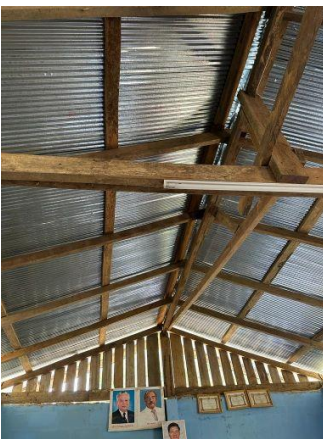
Roof not leaking now – another project
